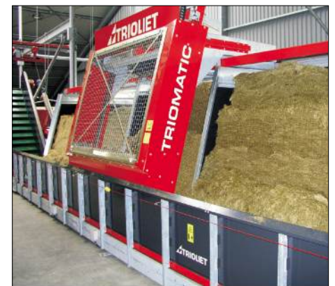
Cross conveyor with electronic weighing system
